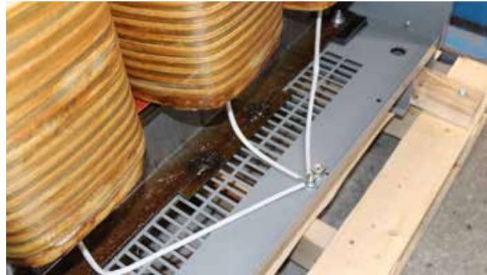
Photo: Electrostatic shield connection to the ground lug
